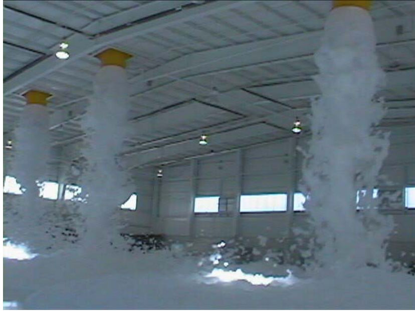
Figure A2.3. Low-Level High-Expansion Ceiling-Mounted Generators' Foam Discharge
